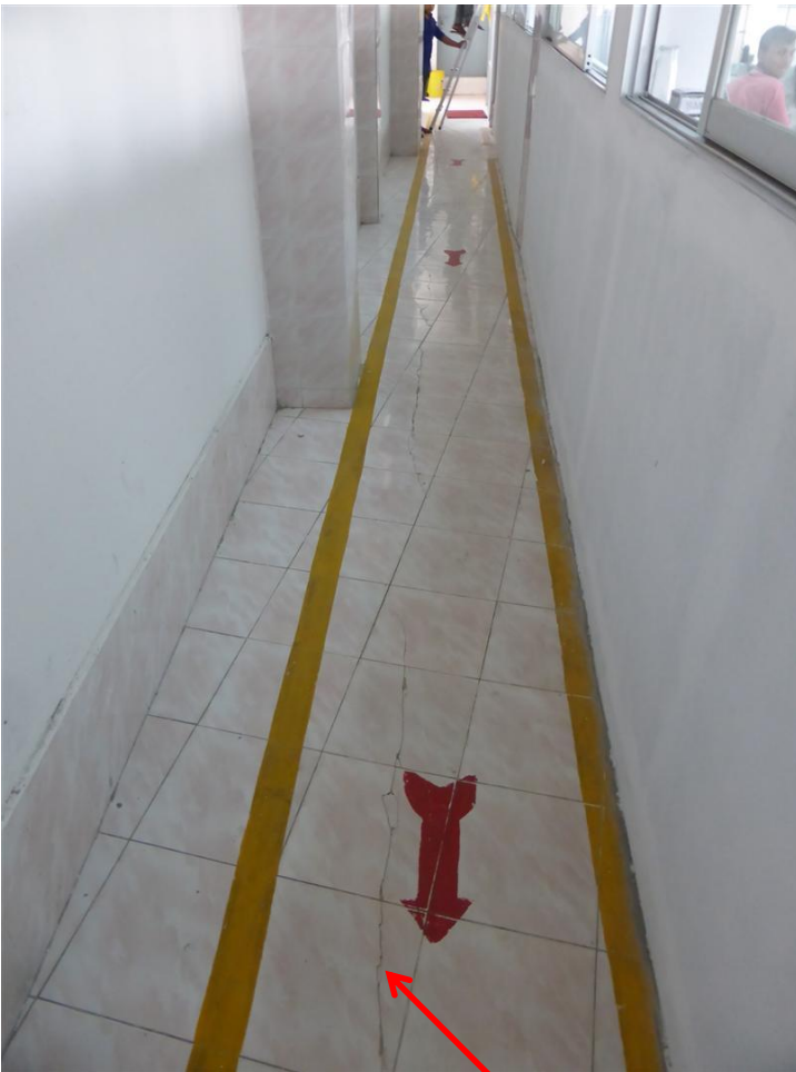
Generator House connected to main factory principally at fourth floor slab. Cracking observed in link slab.
