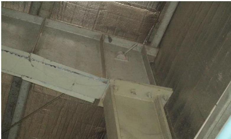
Improper welding was observed in retrofitting location on rafter on various location
