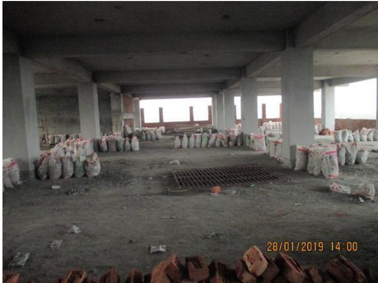
Stack of construction debris on 5 th floor
